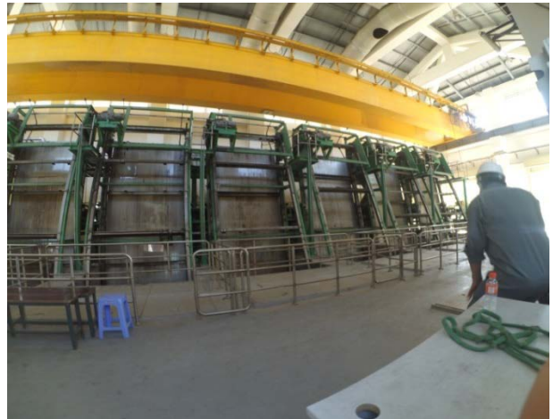
Fig. 2 Song Sai Gon Pumping station
